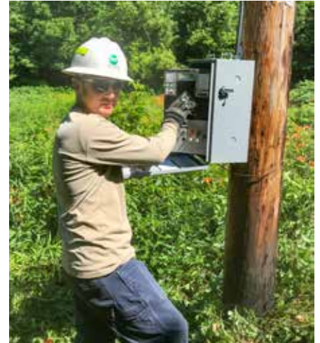
Jackson Energy 1st Class Line Technician, Sean Evans, programs a voltage regulator. Photo: Terry Isaacs
