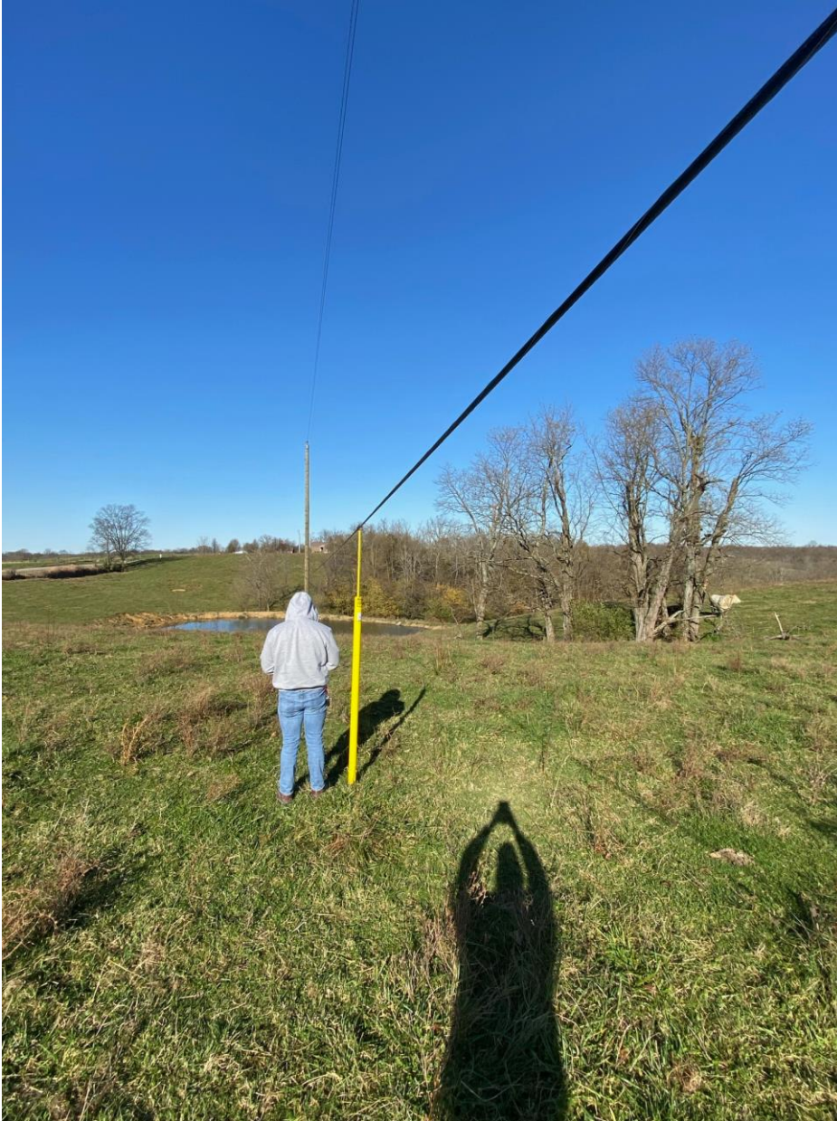
Figure 6 – Communications attachment appears to not be pulled to proper tension causing low midspan height.
